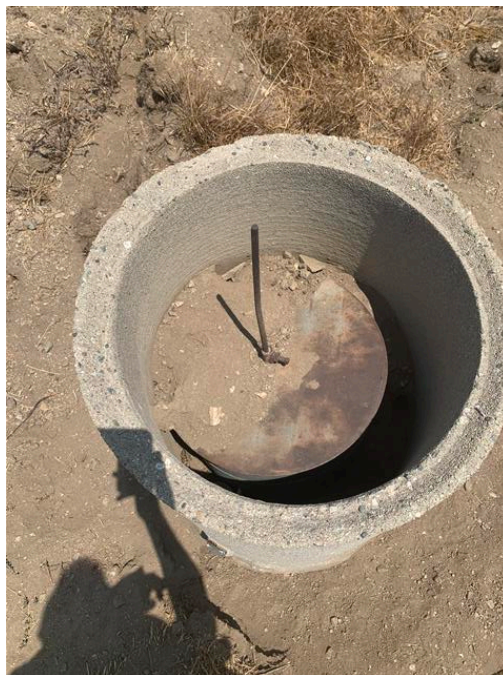
Photo #4 Inside view of irrigation riser located in the central-eastern portion of the Property.
